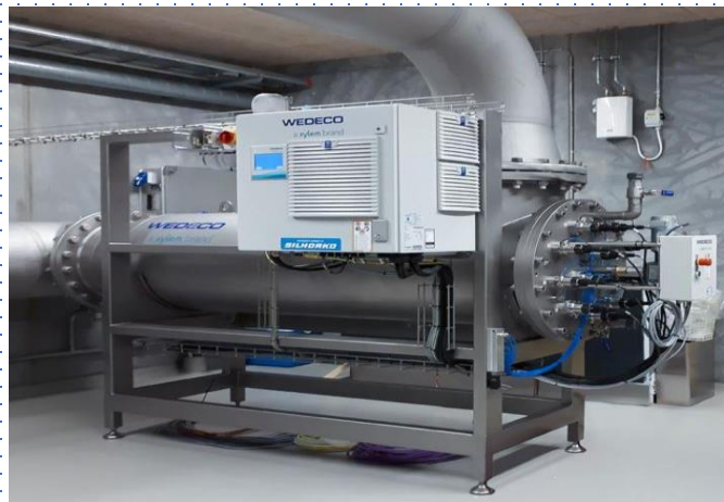
Ultraviolet water disinfection system
